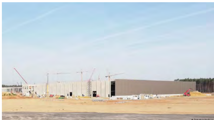
With a final building permit not yet there, Tesla hasn't wasted any time to make its Gigafactory outside Berlin take shape.
